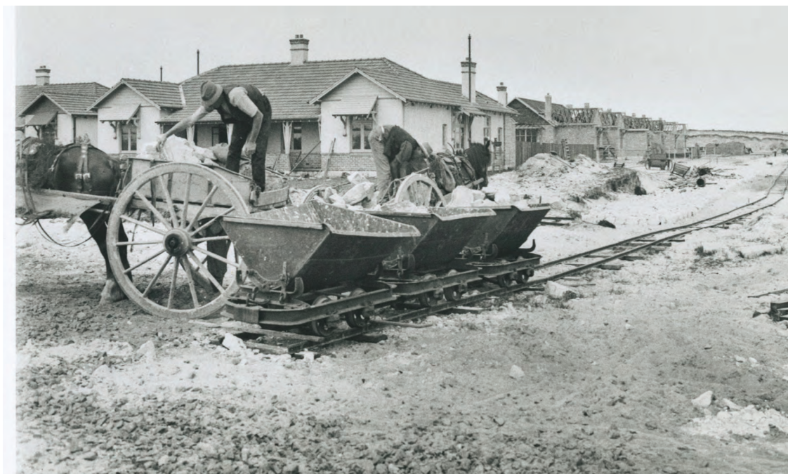
Fig 4.5.8 (below) Constructing Dacey Garden Suburb, c.1916 Astrolabe Road, looking south. (NSW State Records; also SLNSW Government Printing Office 1-30348) also available online at http://trove.nla.gov.au/work/209673513 )
